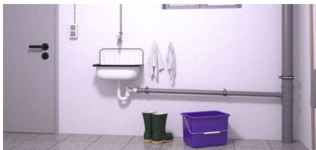
Washbasins with odour traps and washing machine connection
