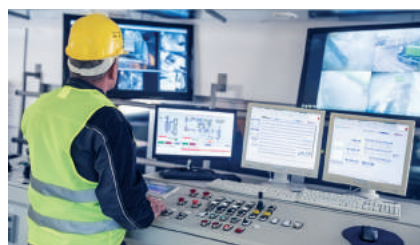
Remote Control Room
